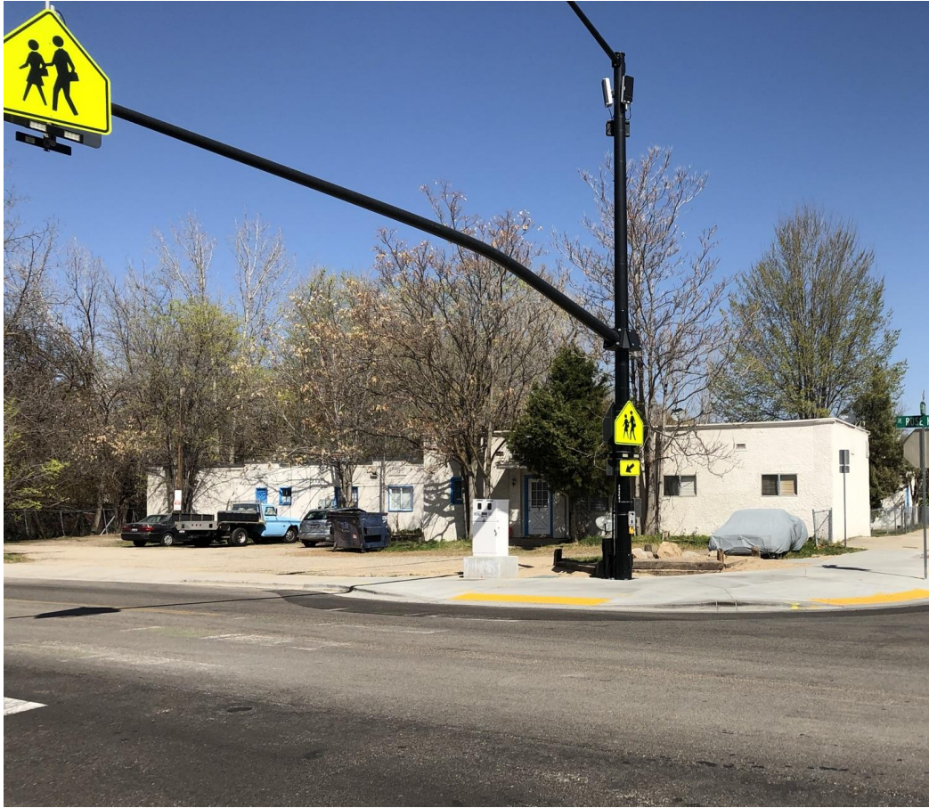
Overhead Rectangular Rapid Flashing Beacon (RRFB)
